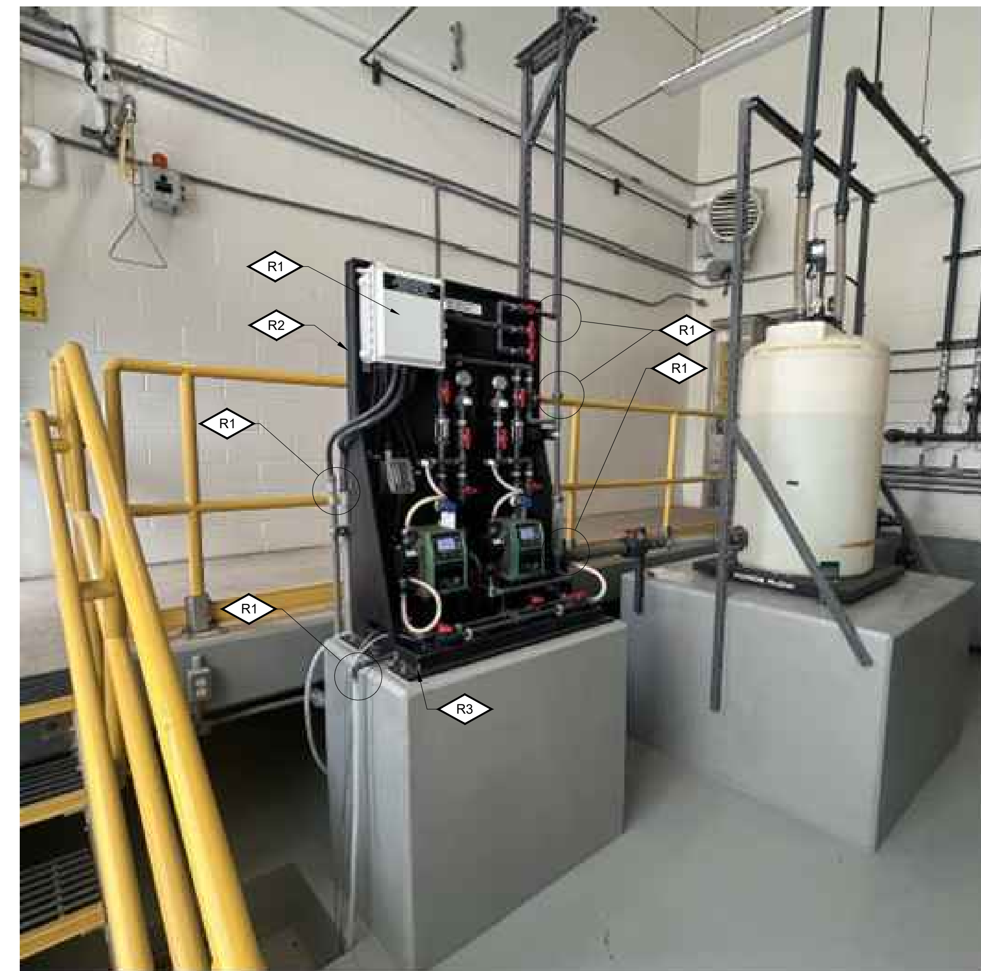
PHOTO: EXISTING BISULFITE METERING PANEL
